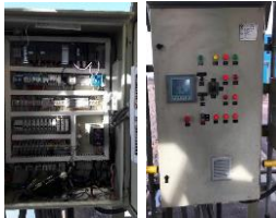
LOCAL CONTROL PANEL
