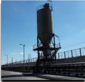
Pellet Lime Coating System
