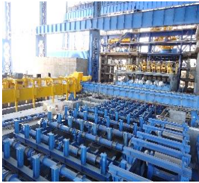
Support Structure for IRT to TCM
