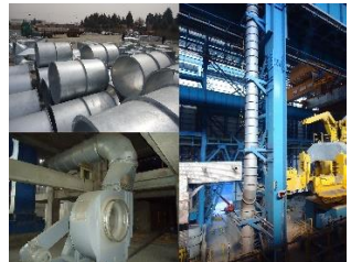
Ductwork Steam Exhauster up to roof
