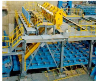
Steel Structure for Rigid Dummy Bar Storage Unit
