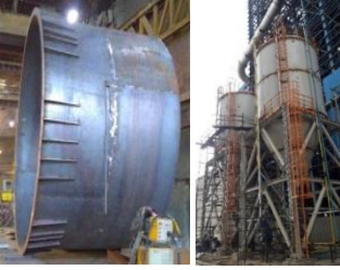
Lime & Carbon Storage Bin
